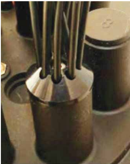
Drop cable sealing
